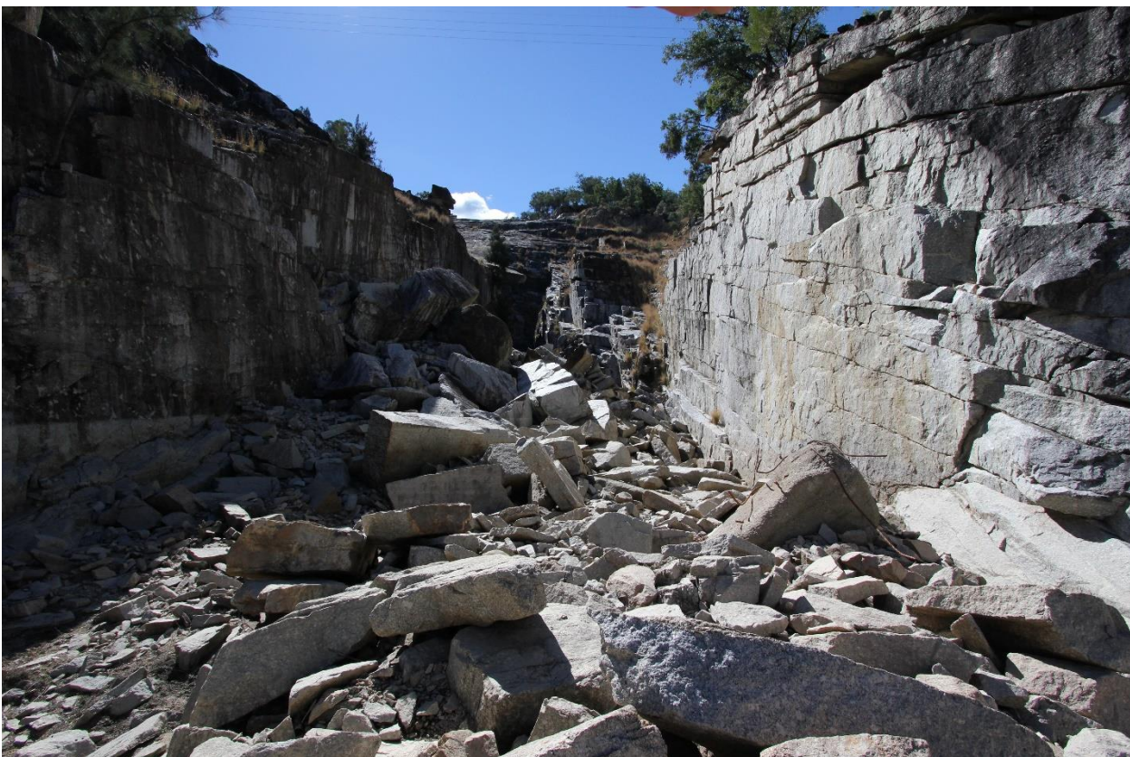
Figure 10. Copeton Dam spillway erosion exacerbated by a fault zone, granite sheet joints and high horizontal in-situ stresses
